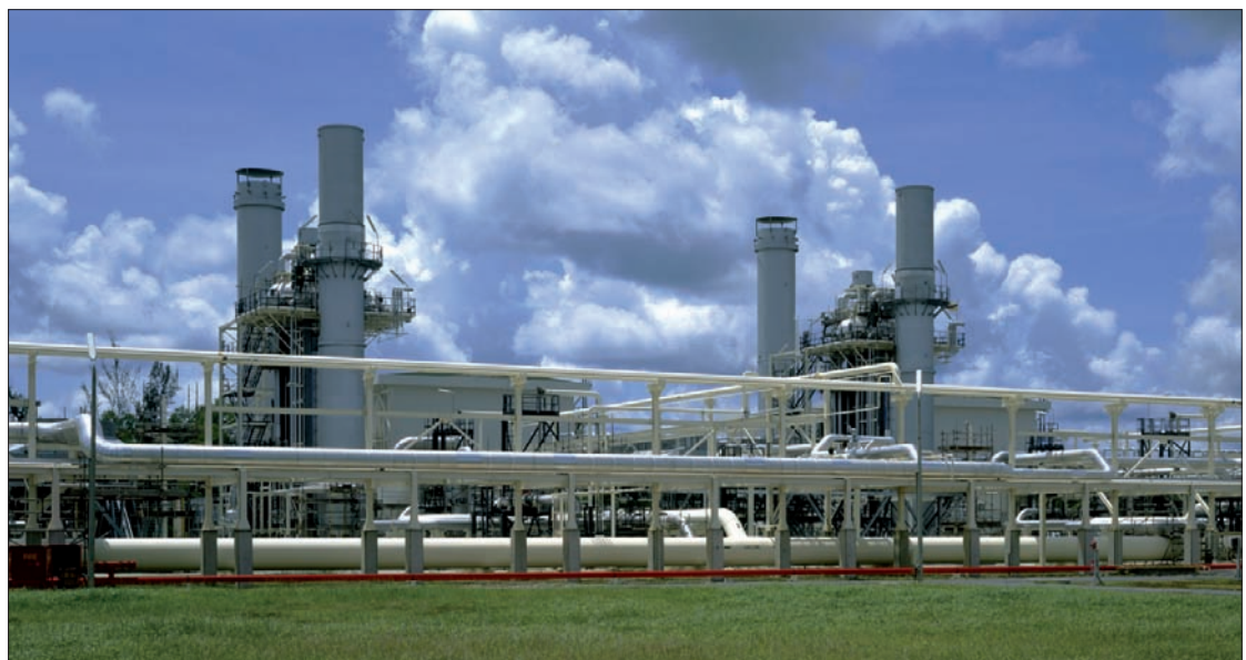
BLNG Liquefaction plant/Gas treatment facility at Lumut, Seria, Brunei Darussalam
