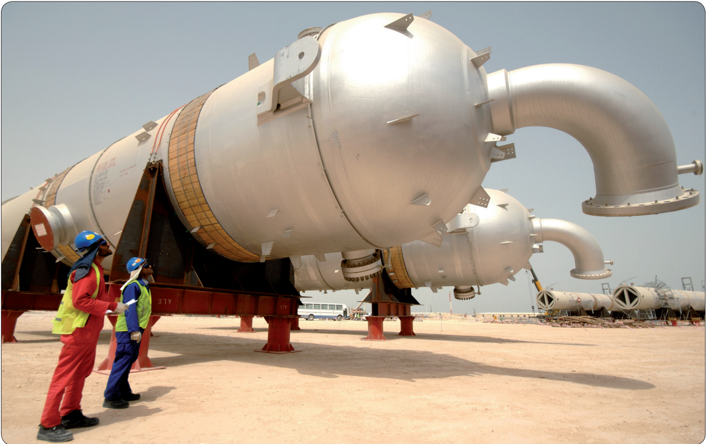
Qatari engineers examine vessels prior to installation at the Qatar Petroleum/Shell-sponsored Pearl GTL plant, Ras Laffan, Qatar
