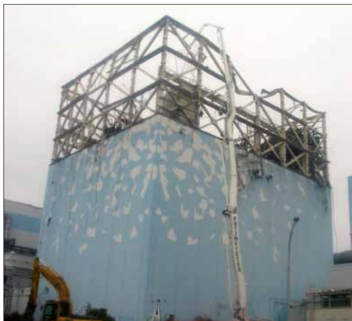
Fukushima Daiichi nuclear power plant Number One reactor building
