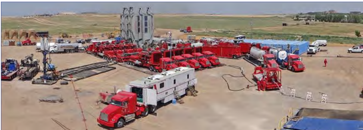
Halliburton’s Frac of the Future™ equipment, including SandCastle® proppant storage units, working in North Dakota
